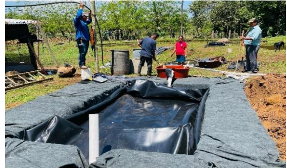
Biodigesters in Santa Cruz de Tojua
